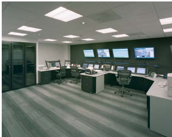
Security Control Room Photo: Jim Roof Creative, Inc.
